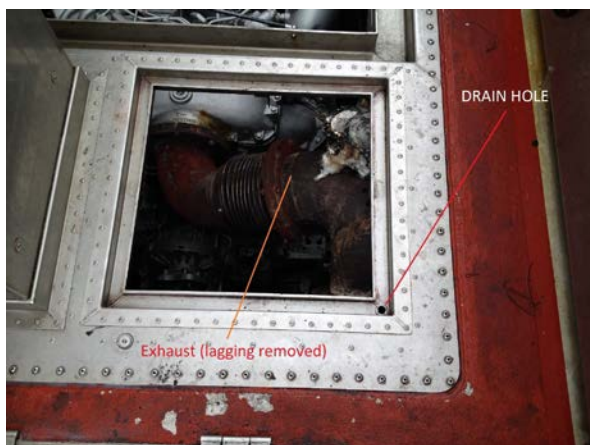
Figure 11: Drain hole from which smoke was sighted
