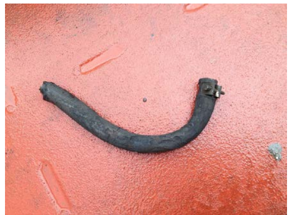
Figure 12: Scorched drain pipe which was immediate cause of fire
