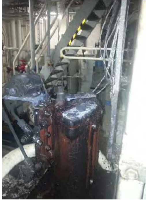
Figure 2: Failed fuel filter unit
