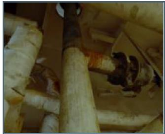
The pipe seen from the lower deck – where the fitter was working
