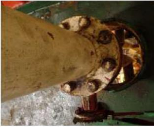
The pipe and the opening through which it had to be lowered. Two helpers were at this location. This was one deck above the fitter's location
