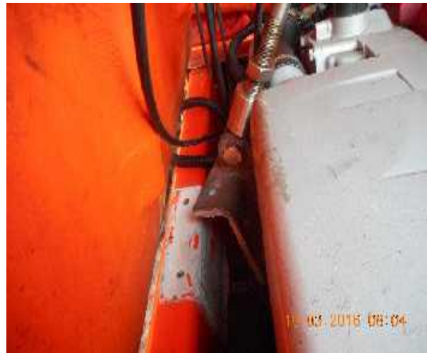
Showing failed starboard load bearing member
