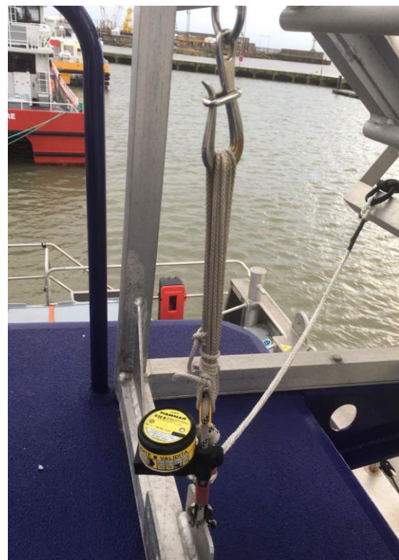
Incorrectly rigged HRU.
