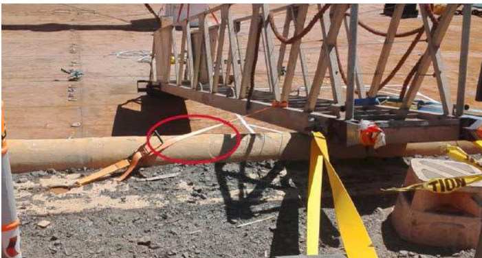
Gangway secured at the high end on the quayside using a cargo strap (cargo strap in direct contact with abrasion point).
