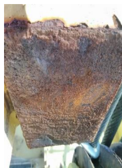
Rust on plate
