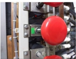
Battery disconnect switch
