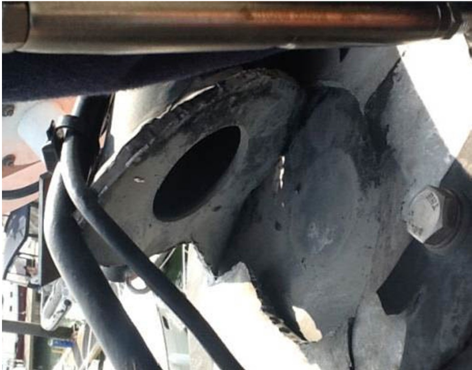
Mast damage following the first incident
