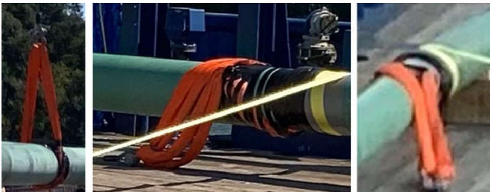
Black duct tape added to “hold” the rigging in place
