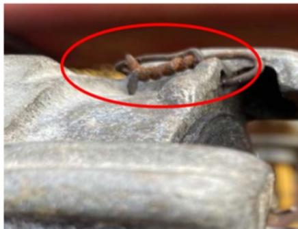
Figure 3 – Baling wire on coupling that released.
