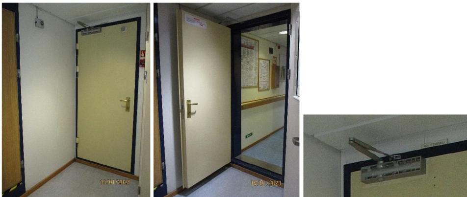
Fire Doors and Closing Mechanism
