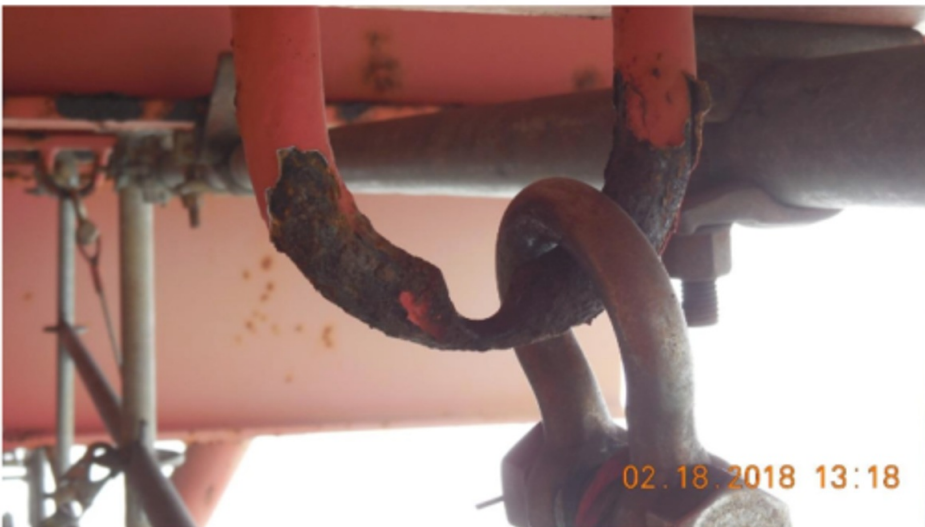
BSEE inspector's photograph of swing rope in place on a Gulf of Mexico facility
