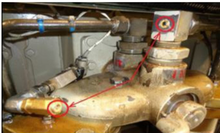
Failed connection as found by duty engineer
