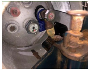
Tank valve and fuel line
