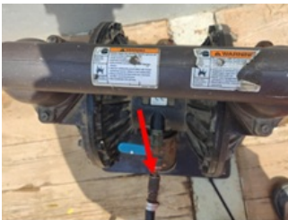
Disconnected hose end connection
