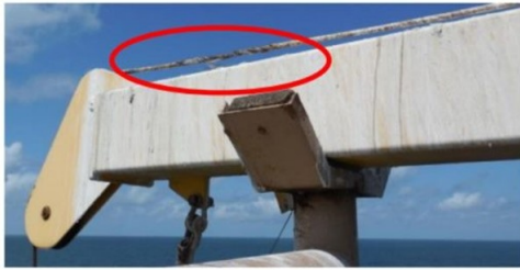
Figure 1 – Corroded crane cable
