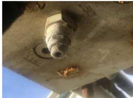
Second valve set incorrectly
