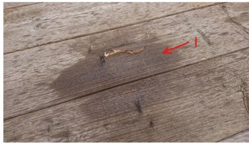
Dents in the wooden deck
