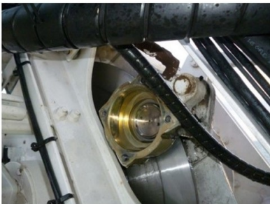
Brake housing showing sheared bolts
