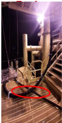
Position of temporary hoses at incident scene
