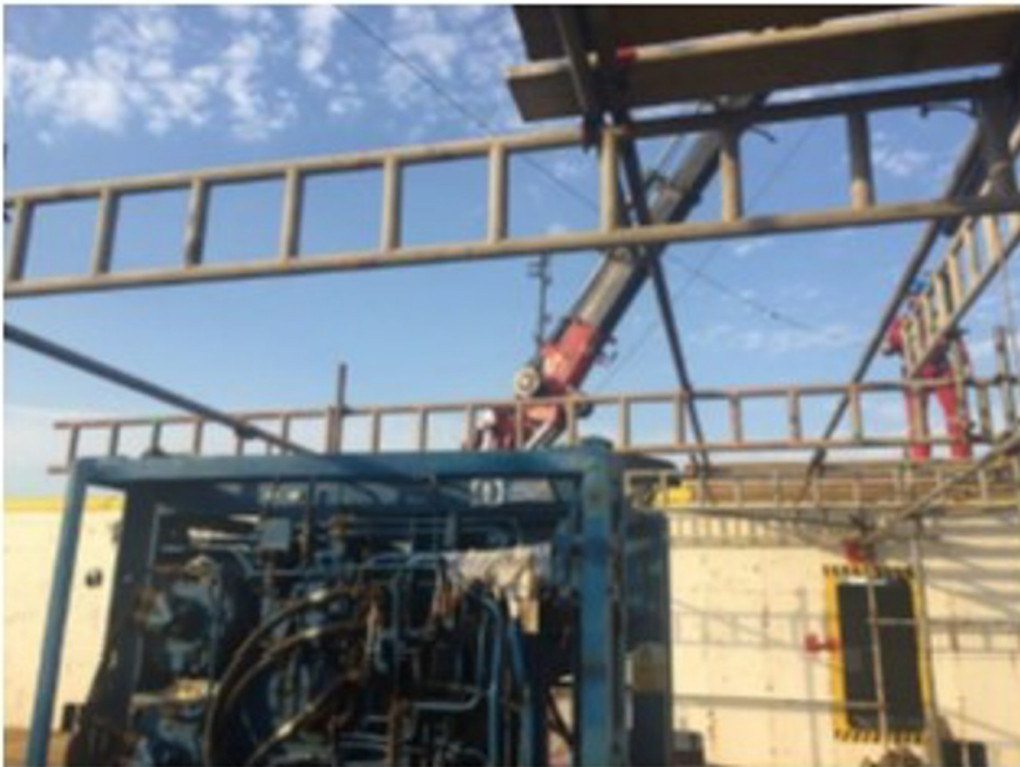
Equipment located on deck
