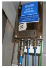
Improper Cable Gland Installation/Modification
