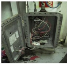
Improperly Modified & Maintained Certified Safe Junction Box
