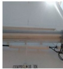
Standing Water in a Certified Safe Flameproof Light Enclosure Indicating Failed Ingress Protection
