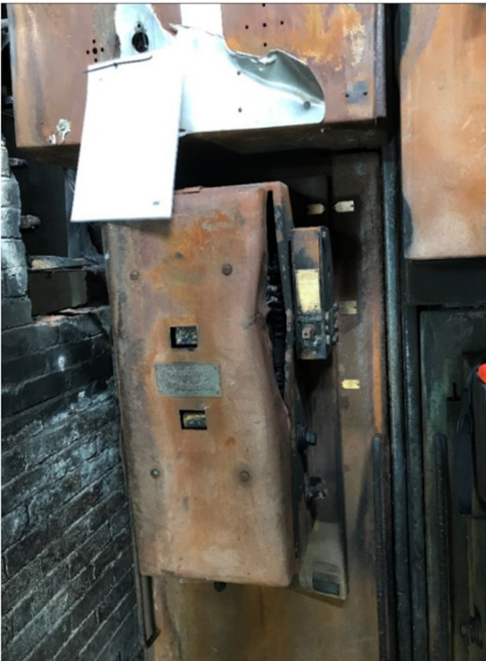
Photograph of the HV oil circuit breaker taken after the catastrophic failure, which resulted in fire and explosion within the substation.
